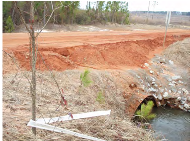
Photo 4: Example of fill placement without BMPs.
