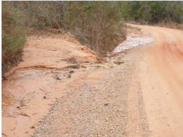
Photo 3: Example of failed “turn-out”.
