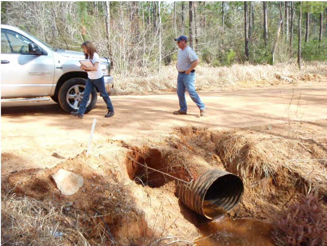
Kilcrease Road near MP 1.8 (12 March 2010).
