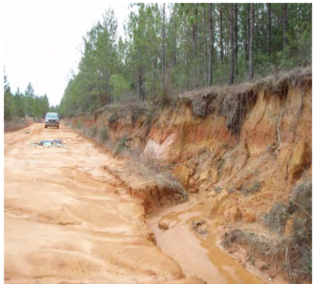
Truck Trail 17 near MP 5.5 (06 February 2010).
