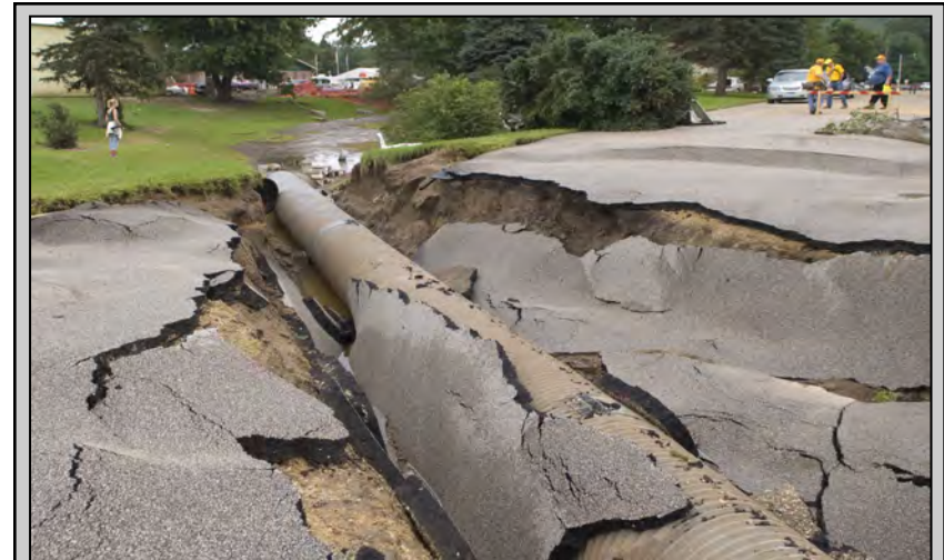
Drainage systems obstructed with trash or other debris can cause an increased risk of flooding since the floodwaters have no place to drain. The increased flooding caused by those obstructed drains can severely undermine the local roadway infrastructure structure, leading to potential health and safety hazards.
