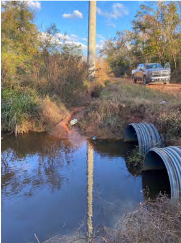
Sediment in Creek
