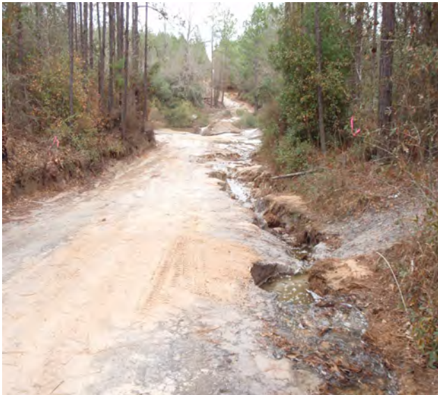
Truck Trail 17 near MP 5.5 (06 February 2010).
