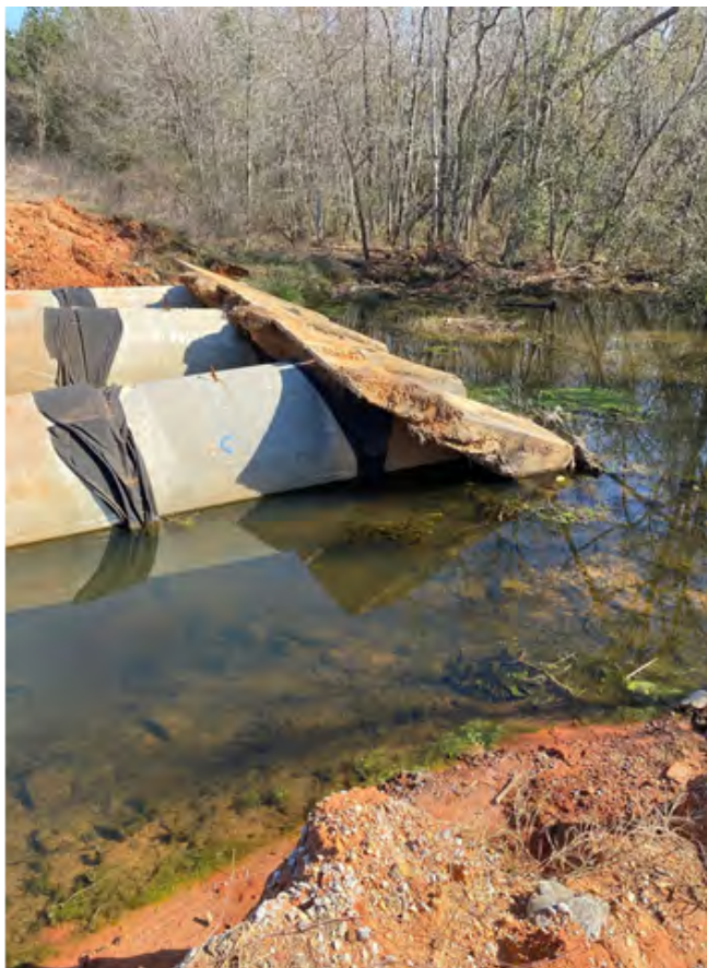
Damage of Culvert System During Hurricane Sally
