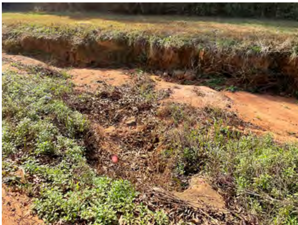
Roadside Right-of-Way Erosion-Flows to Channel
