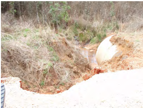
Photo 5: Lack of adequate outlet protection.
