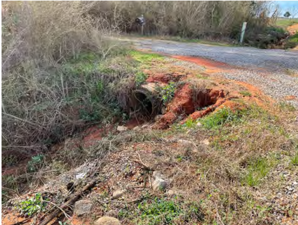
Erosion Near Road Culvert Flows to Wetlands and Stream
