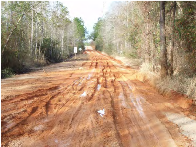
Truck Trail 17 near MP 1.0 (06 February 2010).
