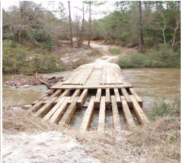
Truck Trail 17 near MP 5.5 (06 February 2010).
