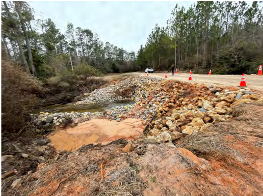
Erosion Noted at Reedy Creek Culvert
