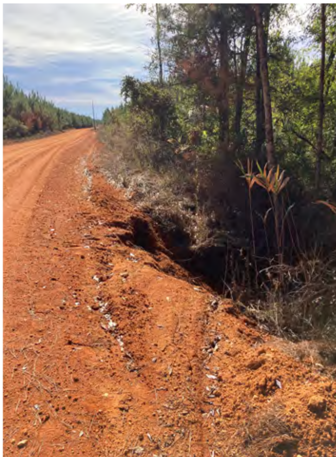
Erosion at Culvert to Creek
