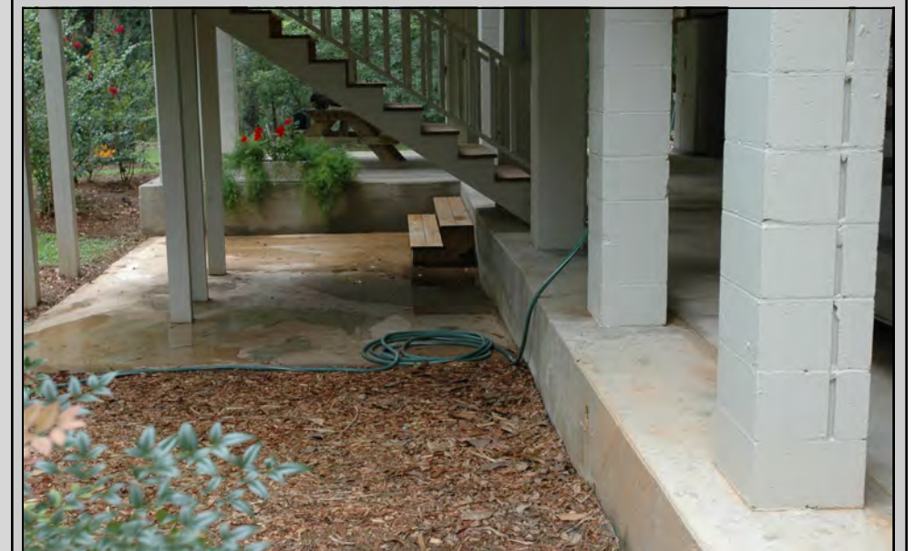
A new 3-foot concrete slab foundation was poured before elevating this house on cinder block piers to mitigate against flooding.
