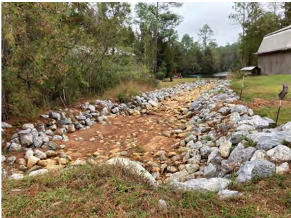
Sediment Noted in Ditch Outfall Discharges to Blackwater River
