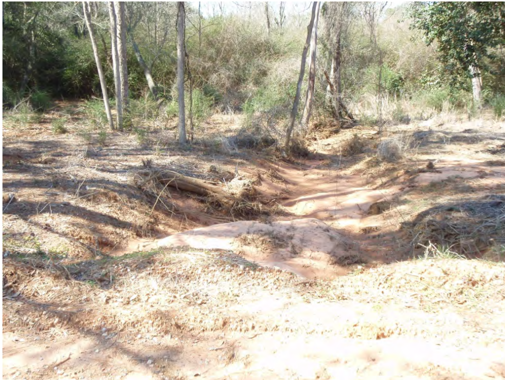
Lipscomb Road near MP 0.2 (20 February 2010).
