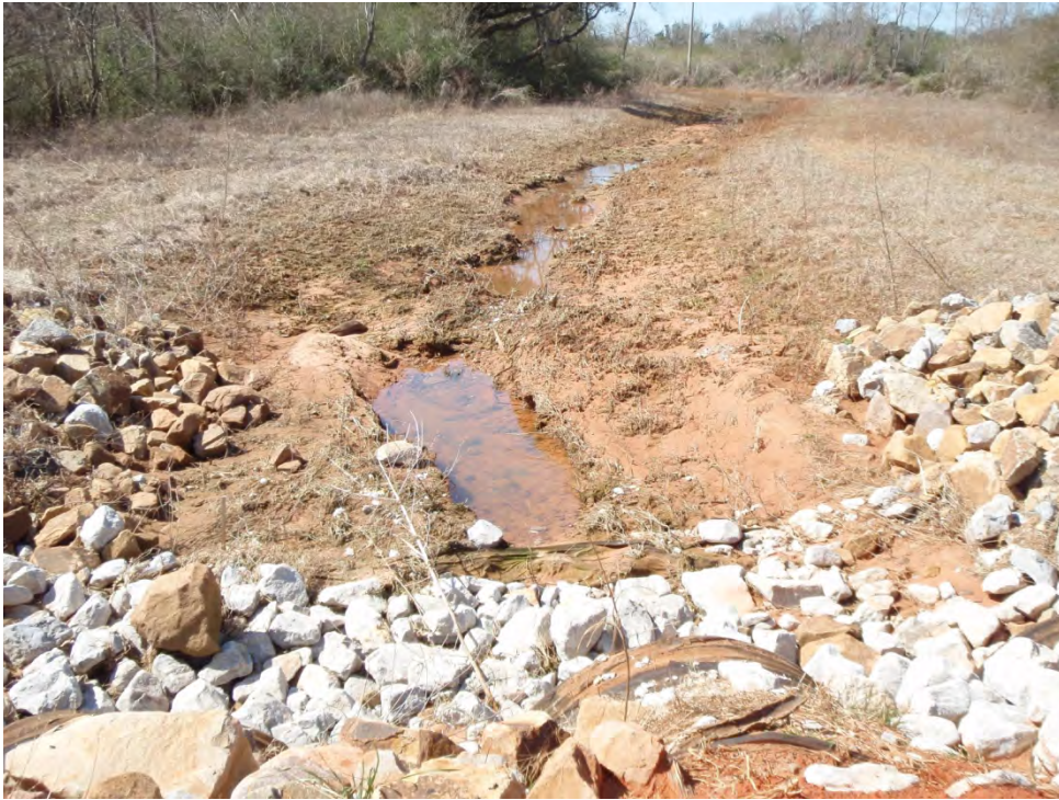
Culvert outlet scour Norris Lane near MP 0.9 (20 February 2010).
