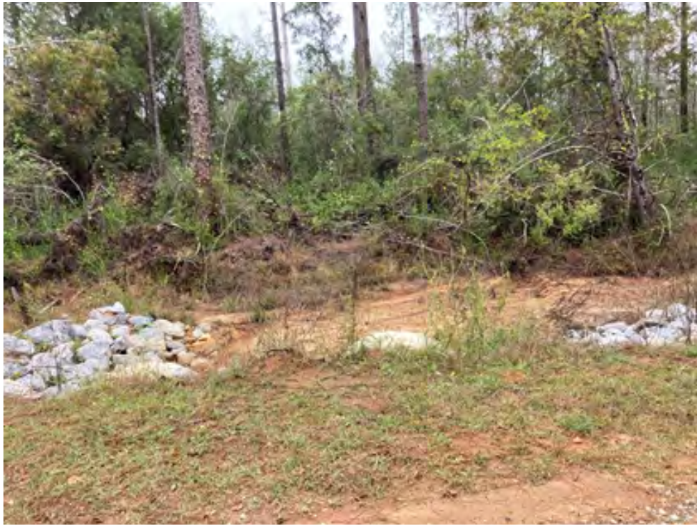
Sediment in Ditch Flows to Blackwater River
