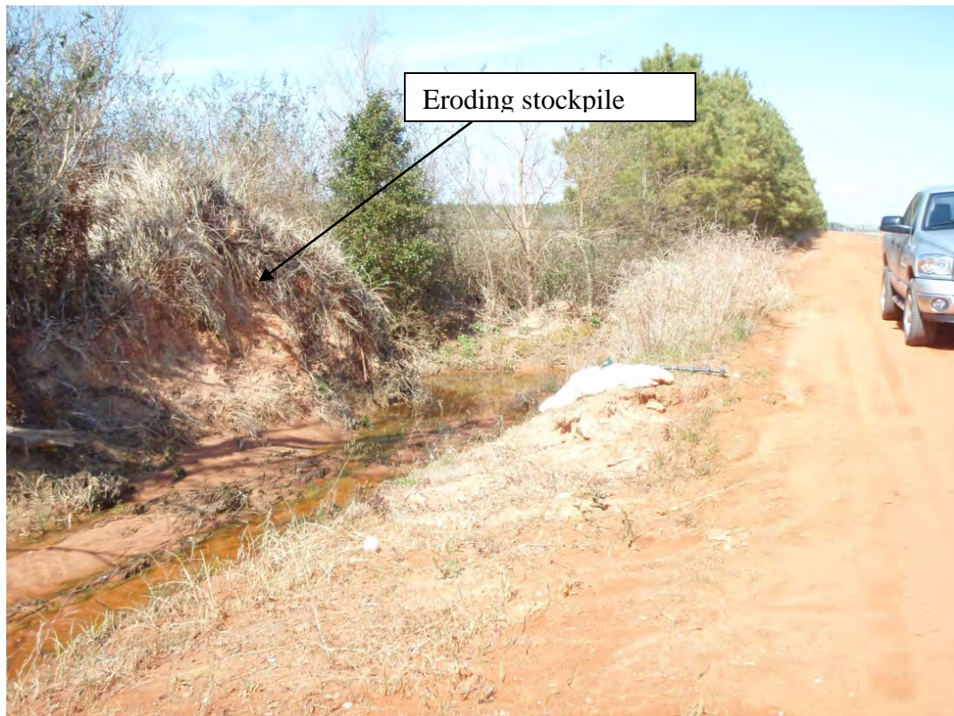
Side-cast stockpile at stream crossing on Norris Lane near MP 0.8 (20 February 2010).
