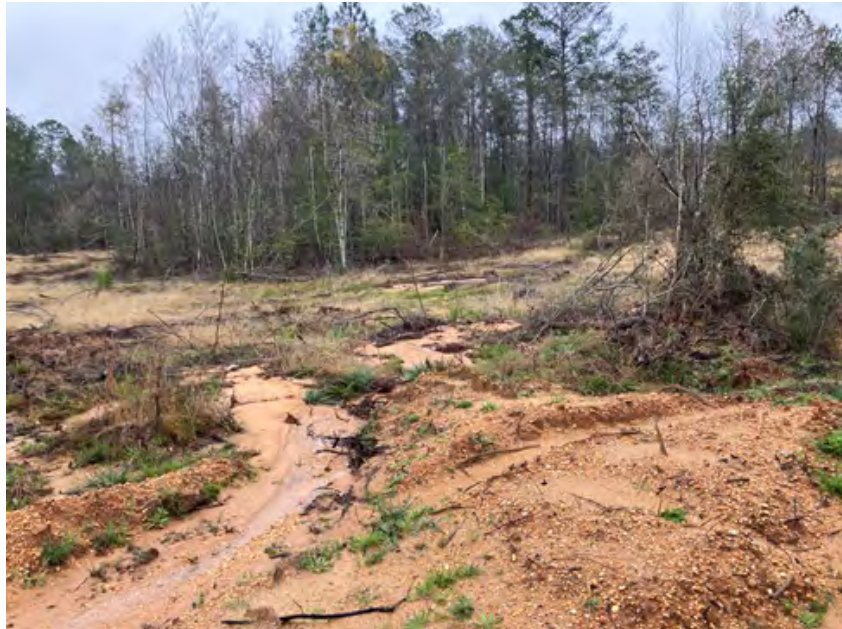
Turnout Discharges to Wetlands
