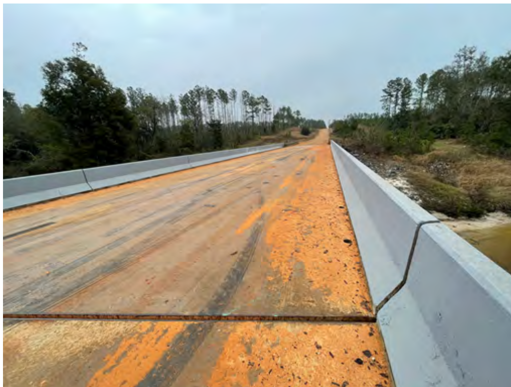
Sediment Noted on Bridge
