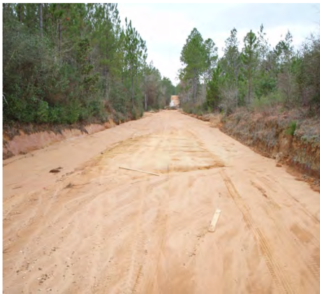
Truck Trail 17 near MP 3.2 (06 February 2010).
