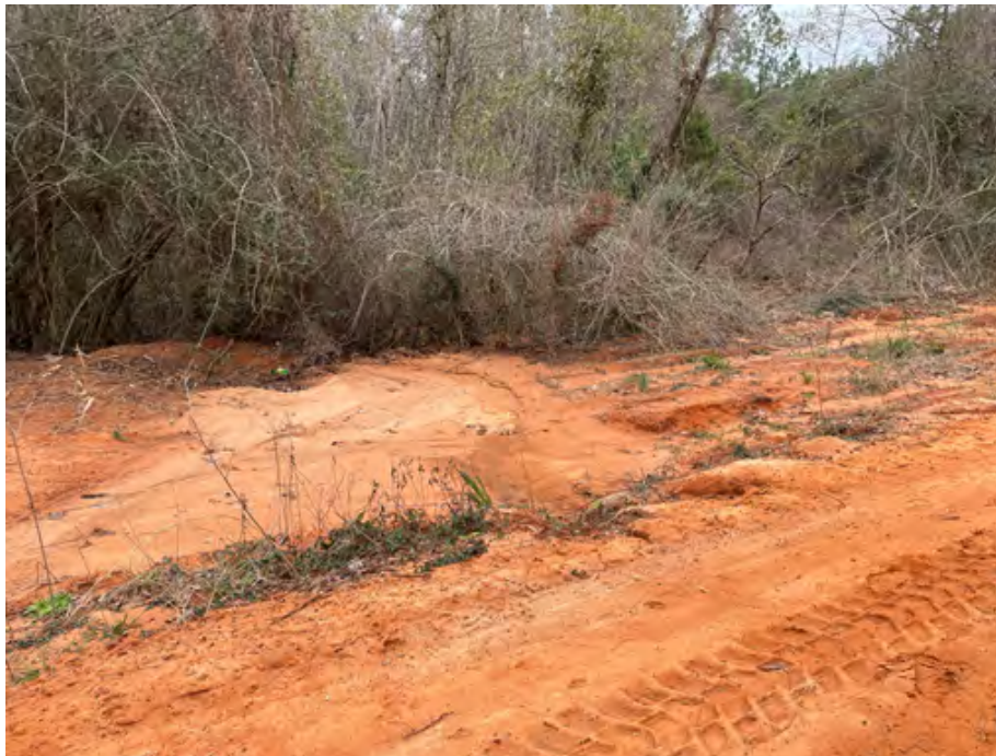
Road Eroding into Wetland Bottom
