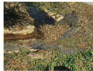
IMG_407-View Upstream Drain Clogged with Debris
