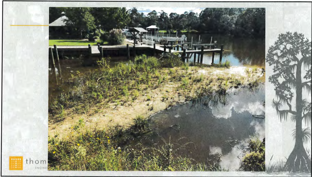
Outfall deposits into Fish River.
