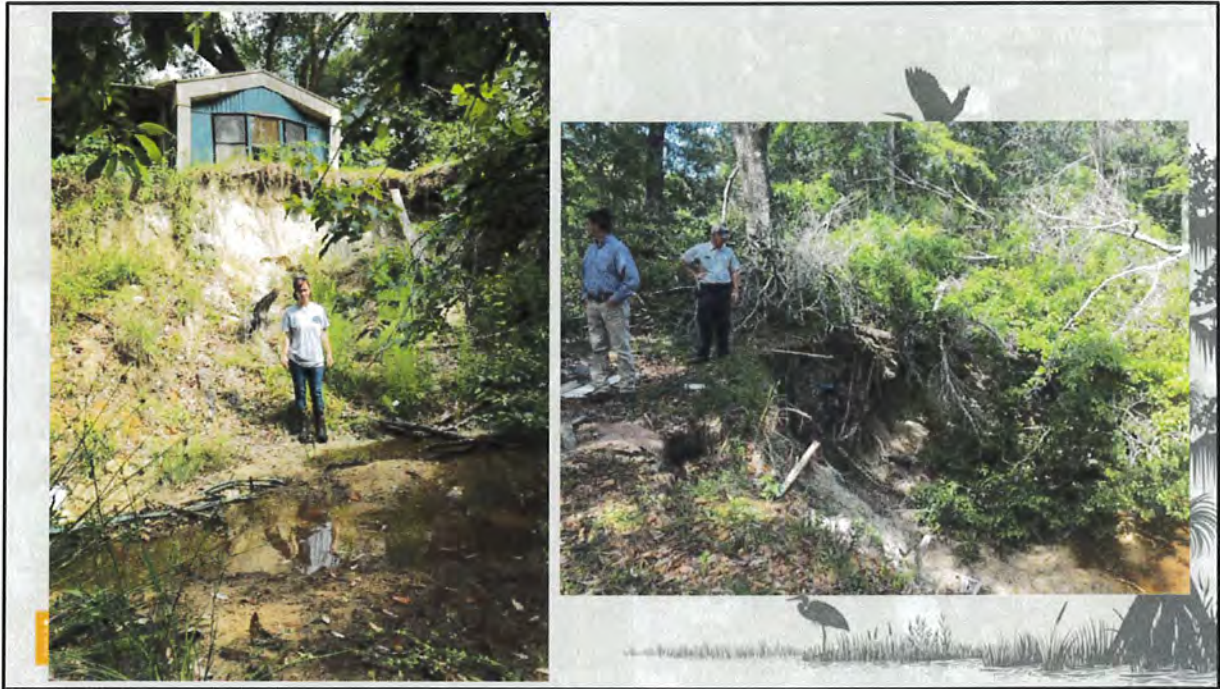
Site condition pre-restoration.
